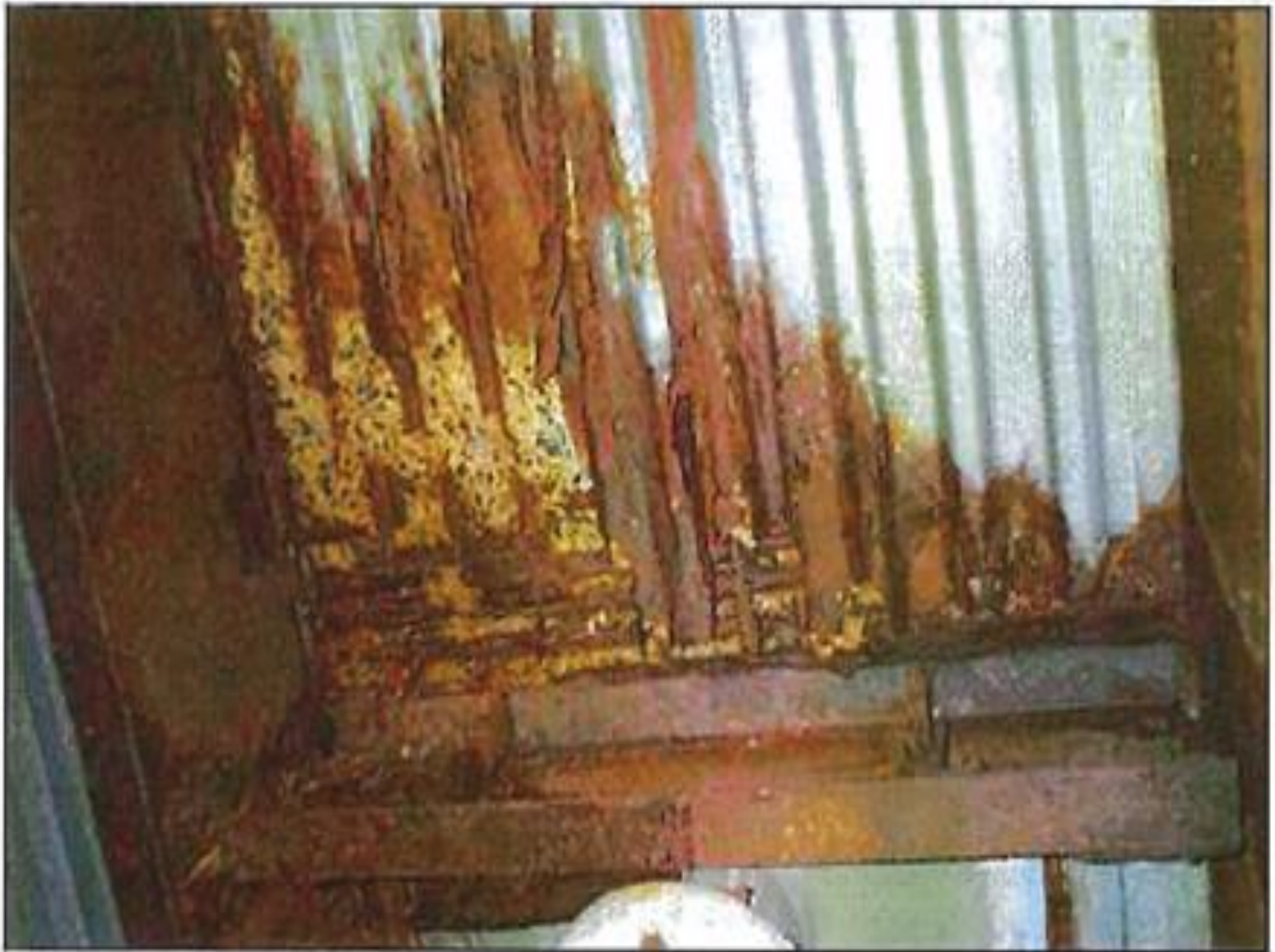
Condition 4 - 100% SIP section loss with underlying concrete exhibiting extensive deterioration and moderate to severe corrosion of exposed reinforcement exhibiting measurable section loss.
